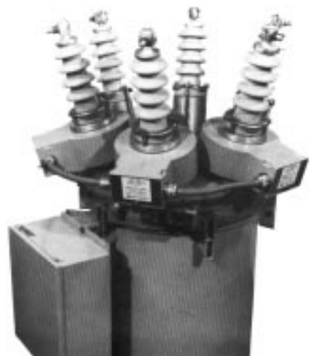
Figure 19. Bushing-current transformer accessory mounted on recloser bushings.
