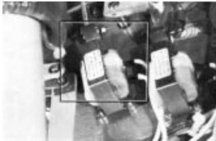
Figure 25. Remote-trip accessory mounted on side of recloser mechanism.
