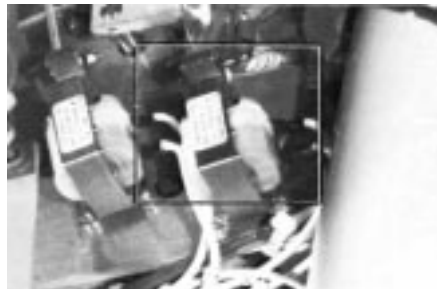
Figure 26. Remote-lockout accessory mounted on side of recloser mechanism.
