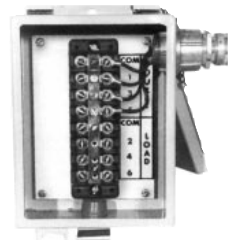
Figure 26. Bushing Current Transformer secondary tap wired to junction box for customer connections. 82086KMA
