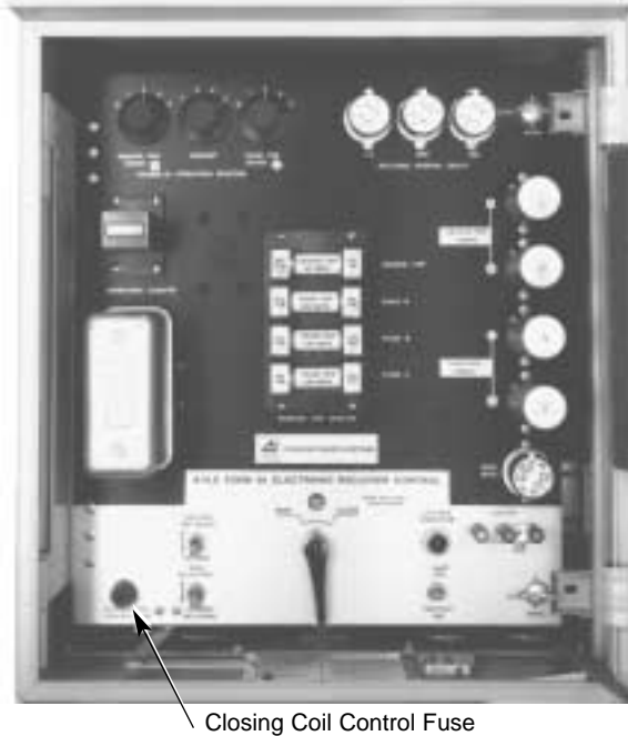
Figure 1. Location of closing coil control fuse.
