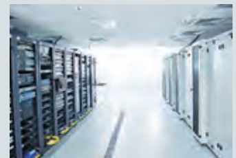
Data center & IT
