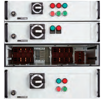
IP2x shielding of the vertical busbar
