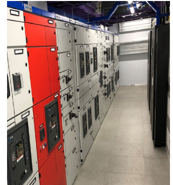
Pictured (left to right): xEnergy, Lithium-ion battery and Power Xpert 9395P UPS
