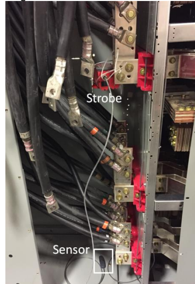
Fig. 7 Strobe in cable compartment
