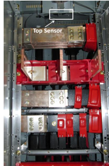
Fig. 3 Bus compartment showing top sensor location
