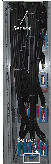
Fig. 4 Cable compartment (top sensor not visible, location noted)
