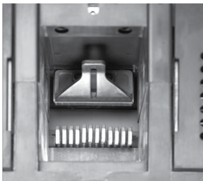
Magnum DS Breaker Contacts (Arc Chutes Removed)
