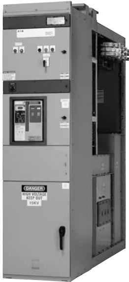
Integrated Unit Substation
