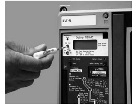
Arcflash Reduction Maintenance System
