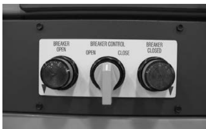
Devices Mounted on Secondary Terminal Compartment Door
