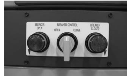
Devices Mounted on Secondary Terminal Compartment Door
