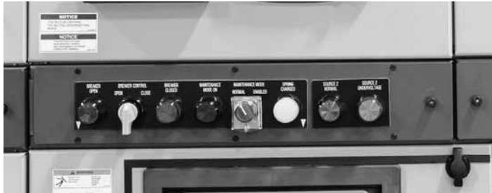
Devices mounted on secondary terminal compartment door
