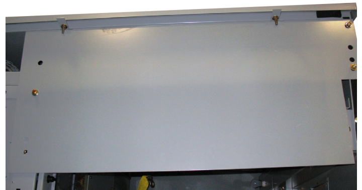
Figure 7. Temporary Shipping Brace on Walk-in Aisleway.
