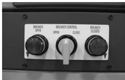
Devices Mounted on Secondary Terminal Compartment Door
