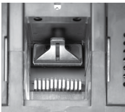
Magnum DS Breaker Contacts (Arc Chutes Removed)
