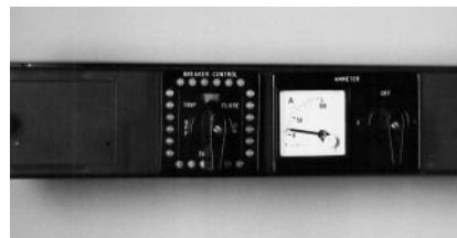
Breaker Control Switch, Ammeter and Switch
