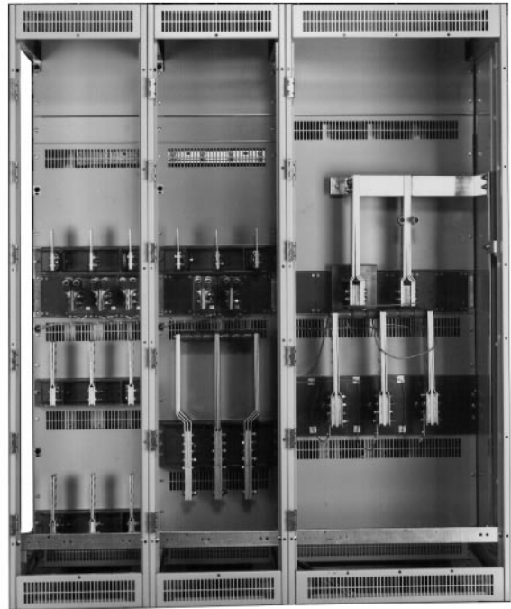
Cable Connection Compartment with Barriers in Place
