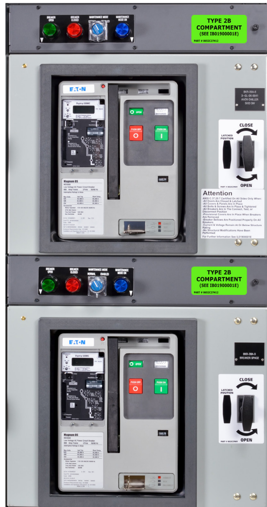
Figure 7. Breaker Bellows On Closed Breaker Door.
