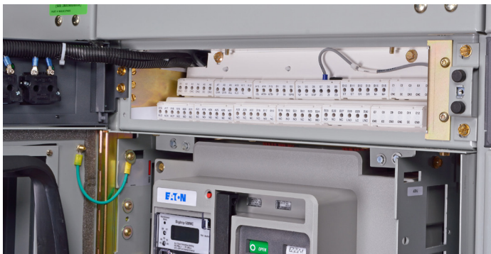
Figure 6. Breaker Bellows On Open Breaker Door.
