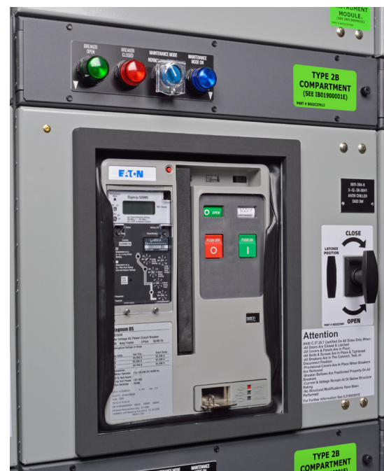
Figure 8. Breaker Bellows In Incorrect Position.
