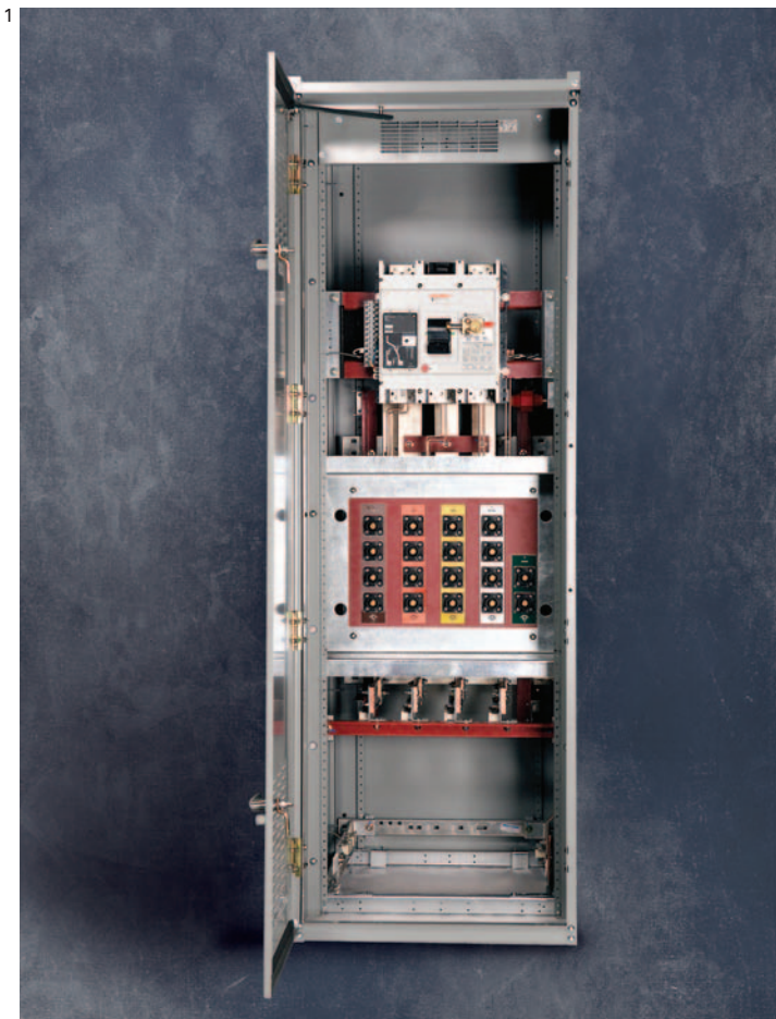
2. Generator Quick Connect Switchboard
