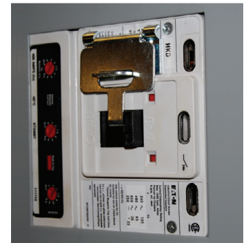
Breaker in ON position.
