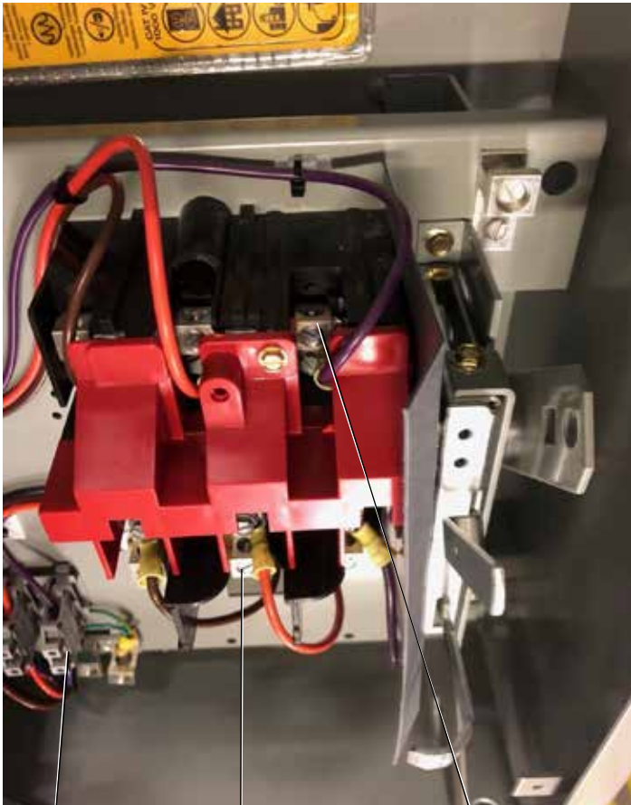
Terminal blocks Voltage indicator wire ring terminals Line side lugs (unwired)
