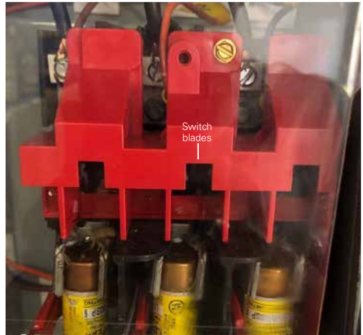
Figure 9. Switch base and fuses.
