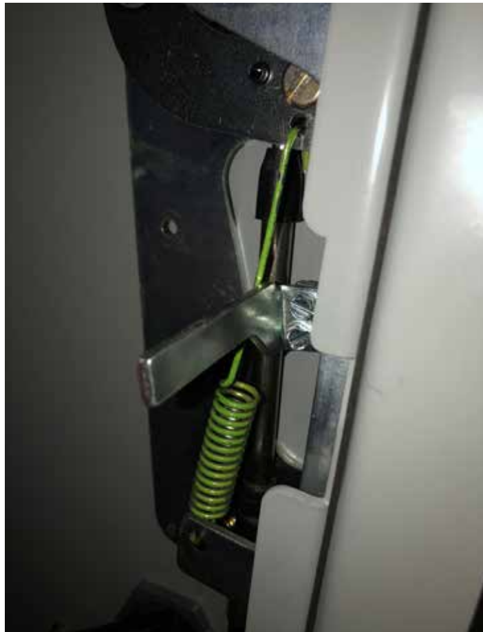
Figure 1. Door interlock mechanism inside control cabinet.
