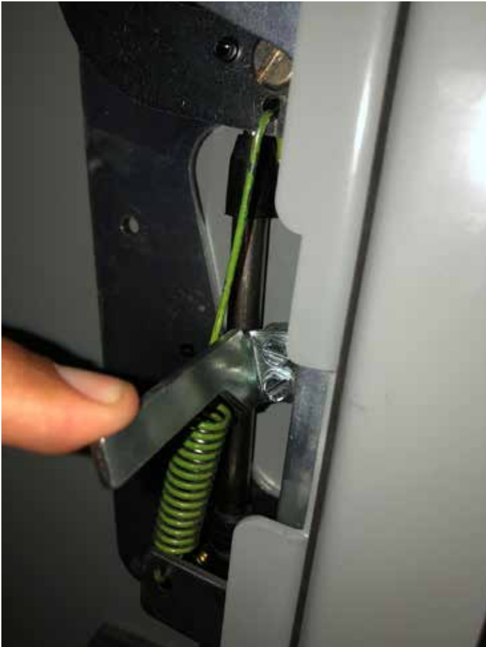
Figure 2. Defeat control cabinet door interlock.
