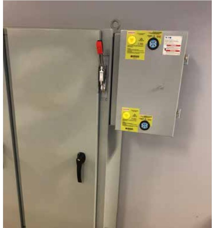
Figure 20. OLI installed on control cabinet with handle in ON position.
