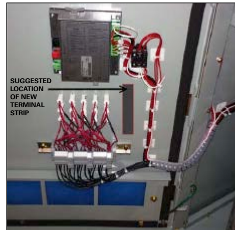
Figure 2. ACX controller and suggested new terminal strip location
