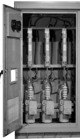
15 kV switched capacitor stage enclosure
