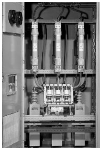
5 kV switched capacitor stage enclosure
