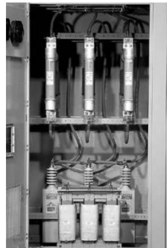
Detuned filter capacitor stage enclosure
