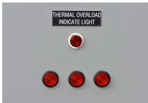
Reactor cabinet thermal overload and cleared fuse indicator lamps
