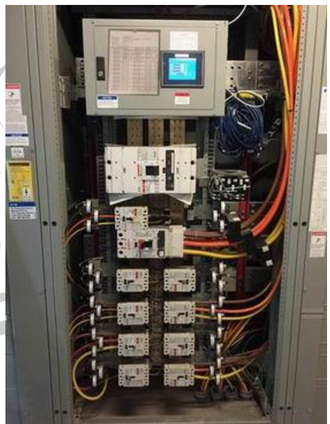
Typical Commercial Switchboard Equipped with PXMP Covers Removed
