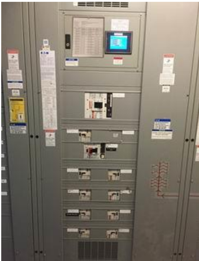
Typical Commercial Switchboard equipped with PXMP
