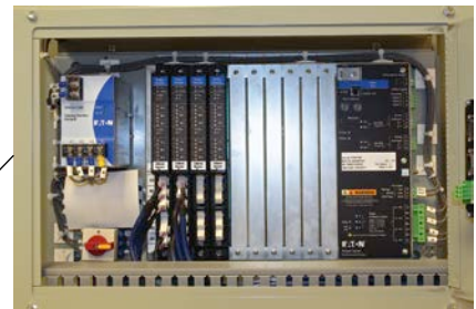
Current sensors are connected to the meter. This will eliminate timely installation cost.
