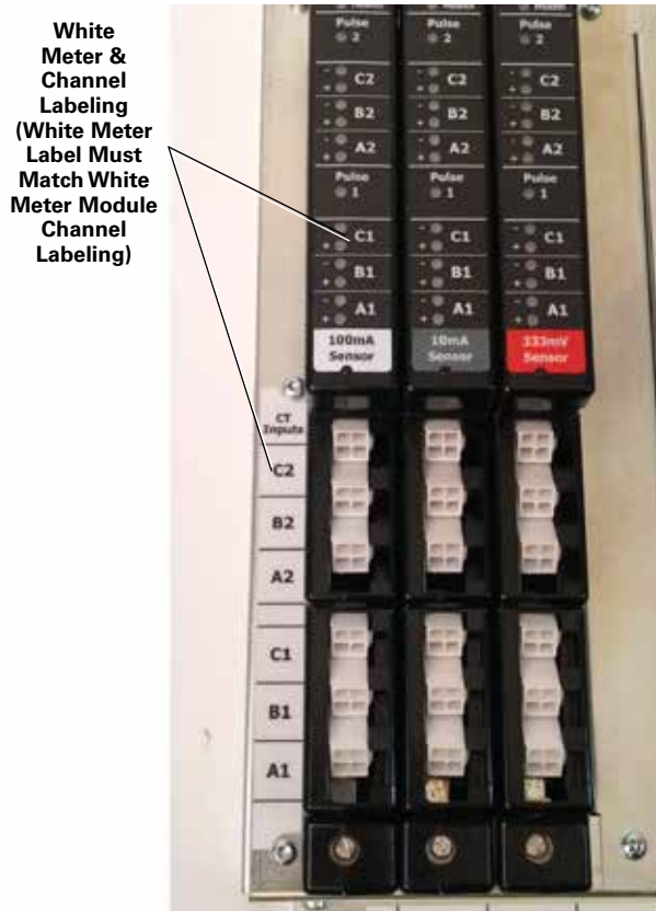
Figure 12. Phase Assignment Label: PXMP-MB Assembly. Note Matching Black/White Meter Base and Meter Module Lens Phase Markings.
