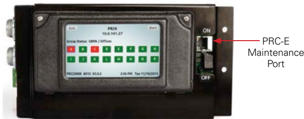
Figure 26. Controller Maintenance Port Connection
