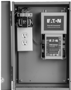
Enclosed PRC5000E Master Controller
