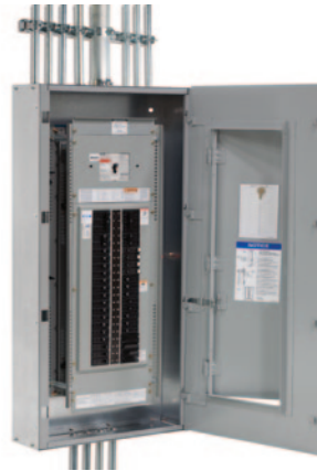
Photo 4. Trim Hanging on Surface Mounted Box
