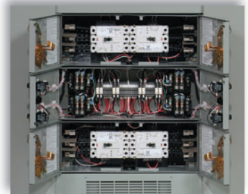
Elevator Control Panelboard
