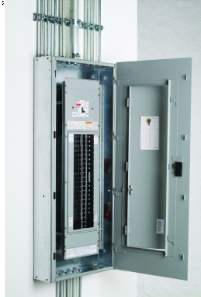
Trim Hanging on Surface Mounted Box
