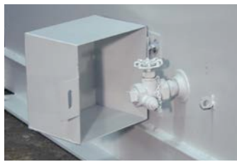
External, pad-lockable drain valve.
