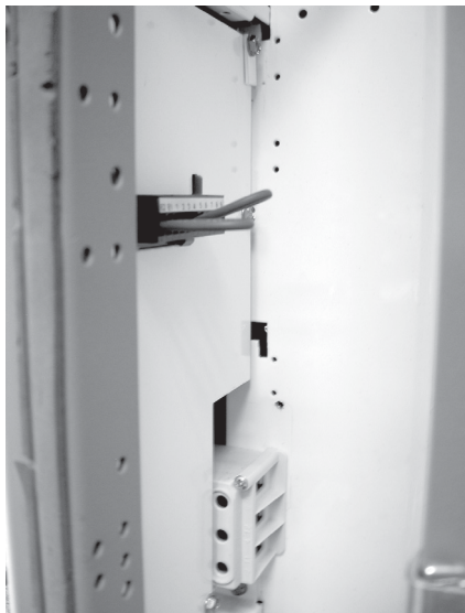
Figure 16. Pull-apart terminal blocks
