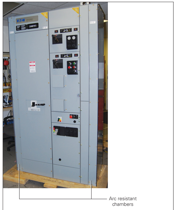
Figure 51. Arc resistant MCC lineup
