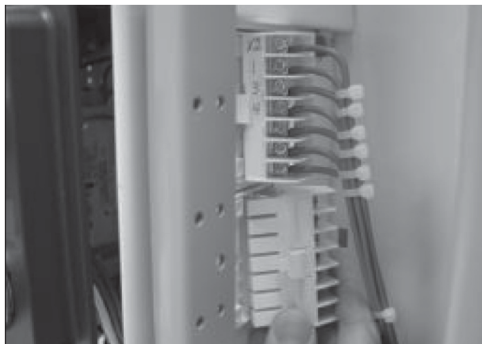
Figure 30. Disengaging pull-apart terminal blocks
