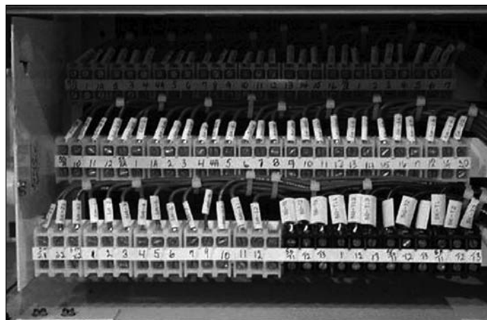
Figure 17. Master terminal block
