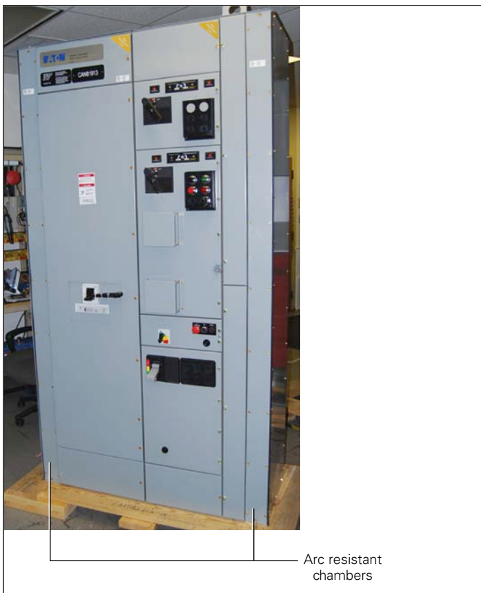
Figure 55. Arc resistant MCC lineup
