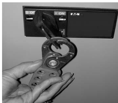
Figure 41. Incorrect application of scissors lock
