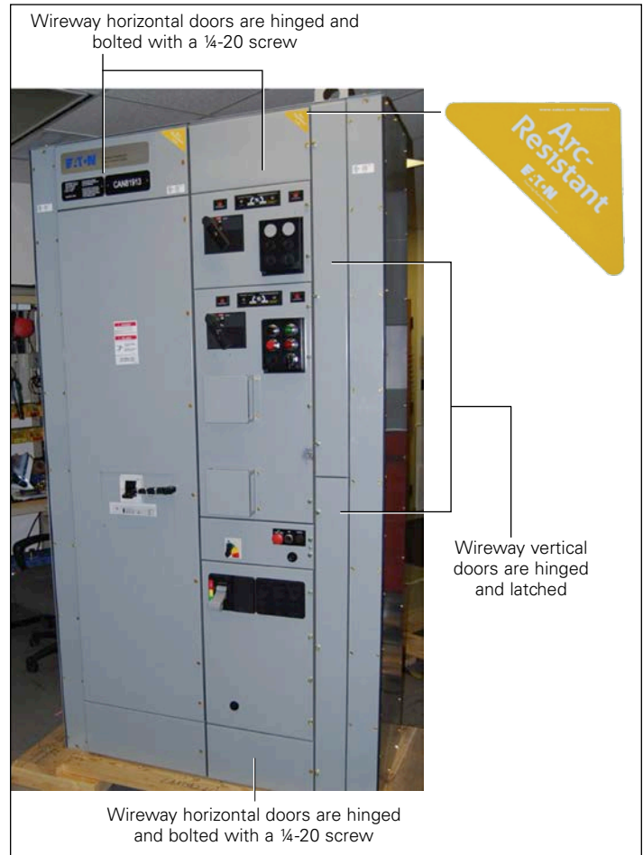
Figure 53. Arc resistant LV MCC—wireway doors and labeling
