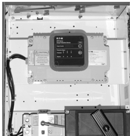
SPD (Surge Protective Device) with Circuit Breaker Disconnect
