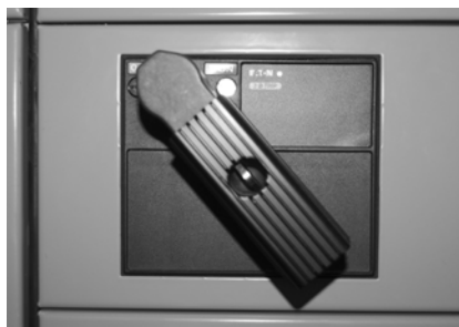
Circuit Breaker Handle Mechanism
