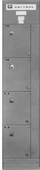
20.00-Inch Wide F10 MCC Structure
