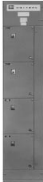
F10 Unitrol Structure
