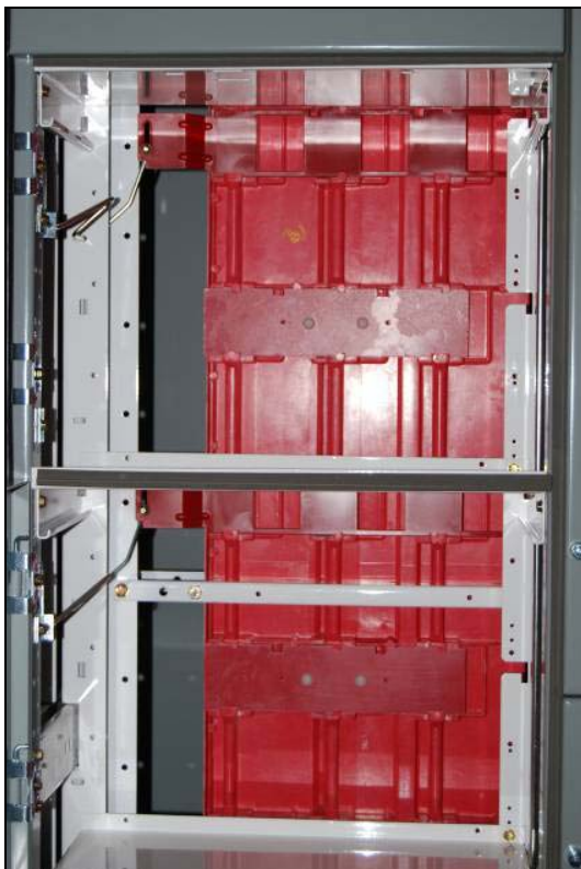
Figure 18. Labyrinth Fully Insulated Vertical Bus.
