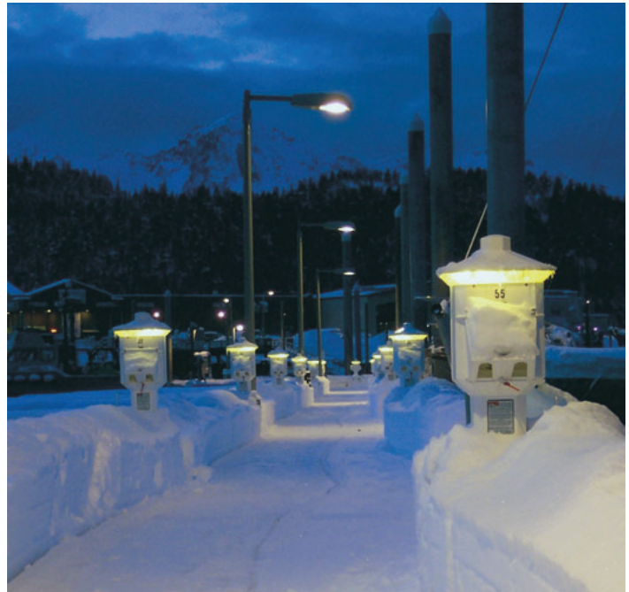
Lighthouse Power Pedestals, Cordova Marina, Alaska
