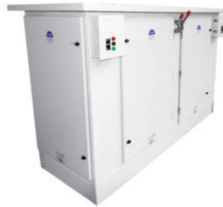
Double Panel Substation
