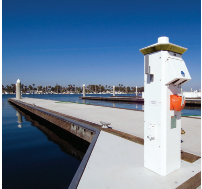
Lighthouse - SS Power Pedestal
