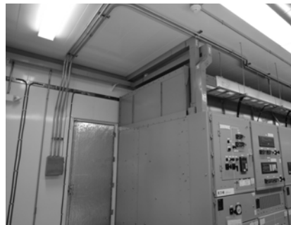
Arc Resistant Switchgear Inside IPA
