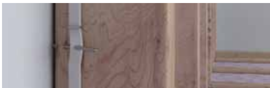
Inadvertent nails can puncture wire behind wall
