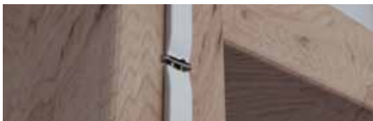
Tight staple can pierce insulation
