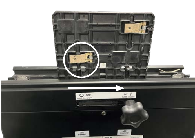
Figure 2. Shows the conductor contacts on the front of the mast open
