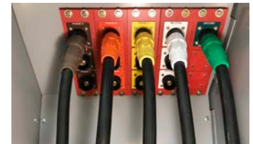
1000 A Cam-Lok power panel with 25% ground ampacity
