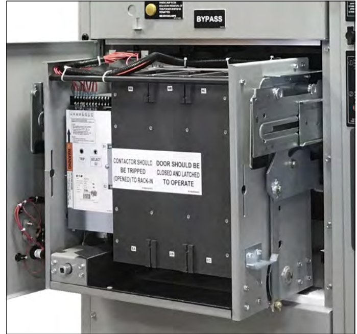
Figure 12. Draw-out Switching Device Extended (to Remove) from the Transfer Switch's Runbacks. ATS or Bypass.
