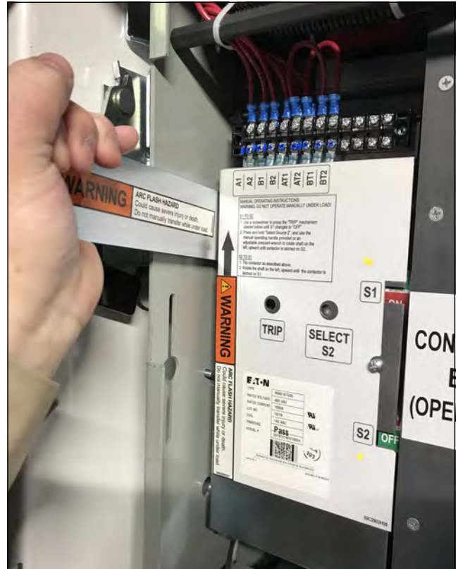
Figure 26. ATS Manual Operating Handle in Use (No Power to Switch).
