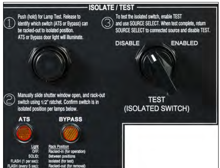
Figure 30. Status Lamps and Controls for Isolation/Test and Removal.
