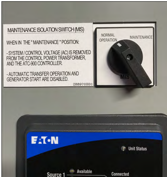
Figure 28. Maintenance Isolation Switch.
