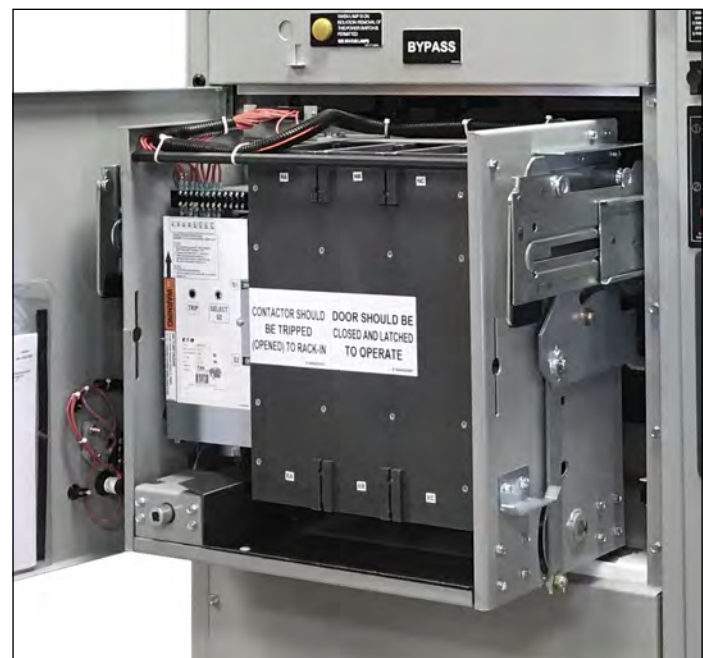
Figure 5. Draw-out Switching Device Extended on Rails for Removal.
