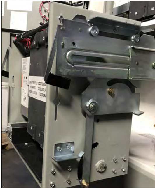
Figure 31. Contactor Racked Out for Removal.
