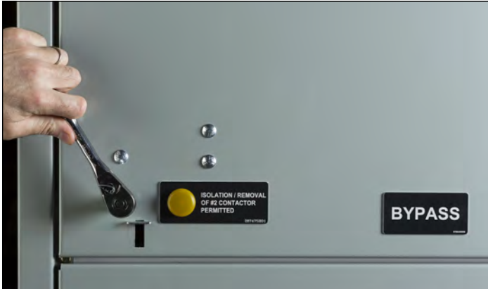
Figure 33. Racked in Contactor Using a Clockwise Ratcheting Motion.
