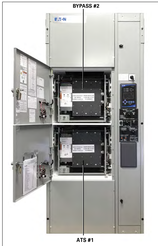
Figure 4. Contactor Devices Installed in the Transfer Switch, Both are Identical.
