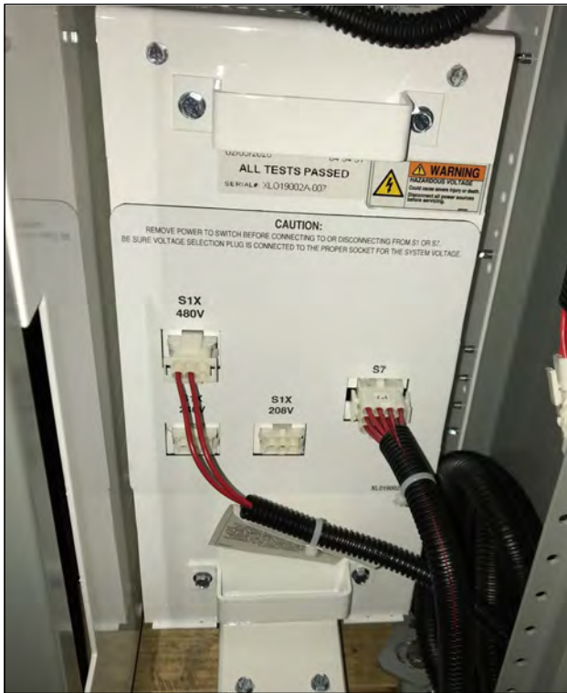
Figure 13. Transformer Voltage Selection Terminals.
