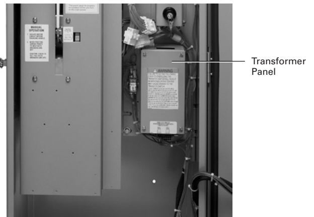
Transformer Panel Location
