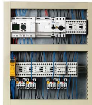
Panel with four traditional starters installed: FVNR, FVR, FVNR with E-stop and FVR with E-stop.
