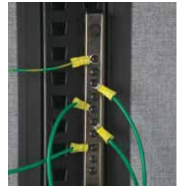
ESD Controls Common point ground bar.
