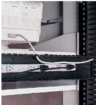
Horizontal and vertical cable management Ducts serve as high-capacity raceways that accept wiring and optional power strips.
