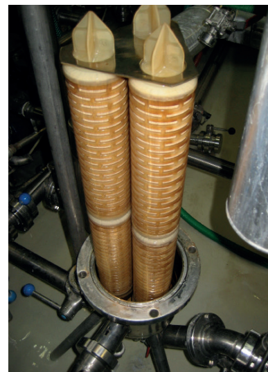
Figure 3: Thick dirt and iron deposits (filter cartridges).
