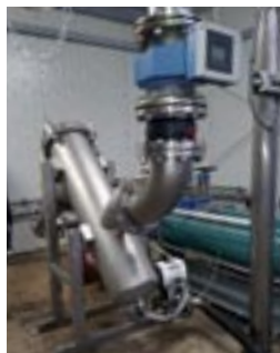
Image 2: At the sewage treatment plant, the fully automatic strainer basket filter replaces a manual solution that costs operations personnel several hours of work per day. © ESB Bocholt
