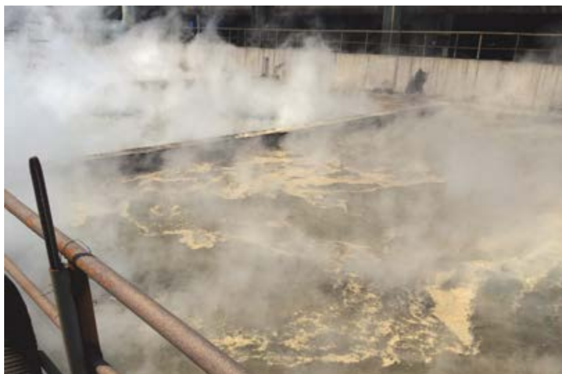
A sink basin with cooling water that is contaminated with iron fragments, sand and mineral particles.
