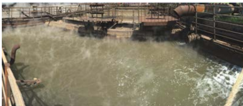
Cooling water after being filtered with the automatic self-cleaning strainer and ready for re-use.
