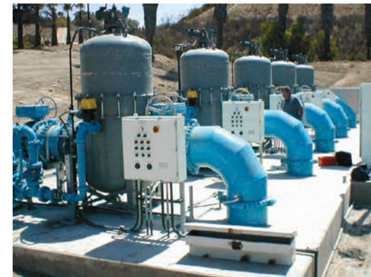
Five 24" Eaton Model 2596 strainers with backwash assist pumps installed at a potable water treatment plant.
