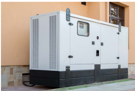
Engine / Generator starting
