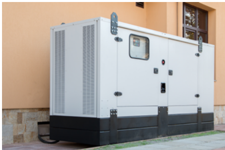
Engine / Generator starting
